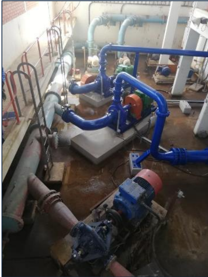
Figure 13.42 Olifantskop Clear Water Pump Station (Umgeni Water 2019).
