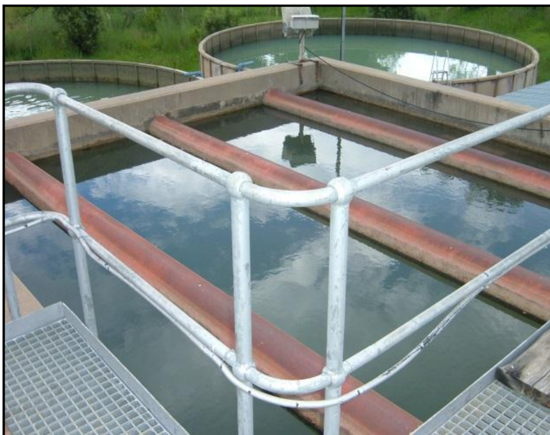
Figure 13.55 Colenso WTP (Umgeni Water 2017)
