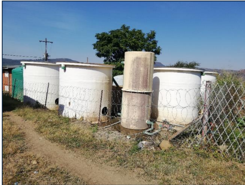
Figure 13.33 Tugela Estates WTP clarifiers (Umgeni Water 2019).
