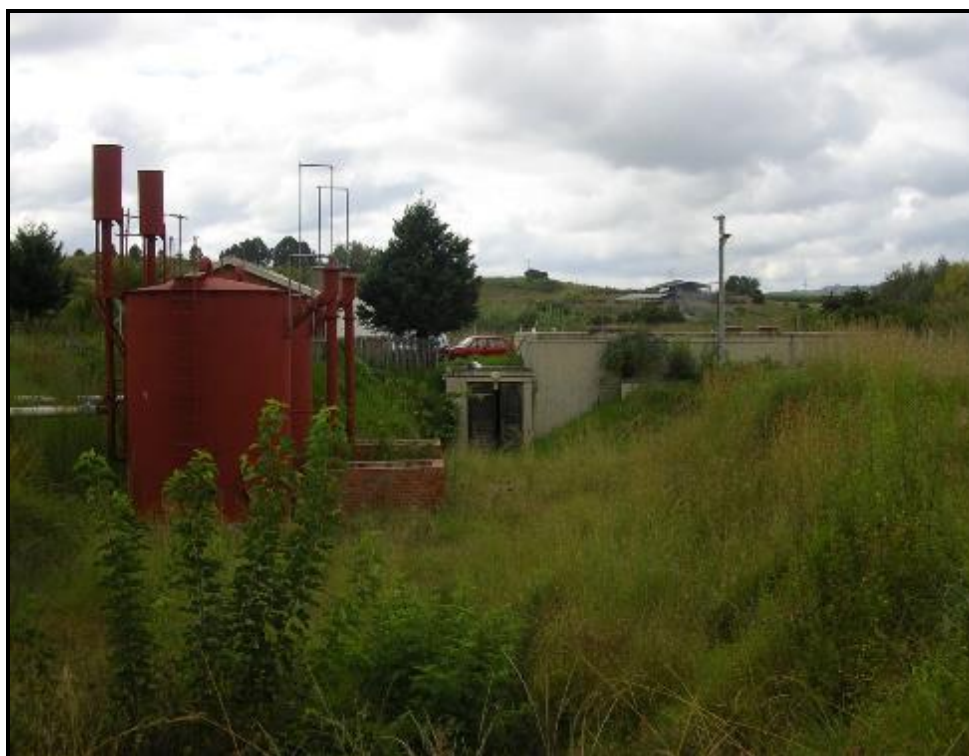
Figure 13.52 Bergville WTP (Bigen Africa, O & M Manual Bergville, 2009)
