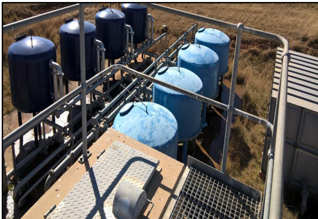
Figure 13.49 Zwelisha Moyeni WTP (Umgeni Water 2017)
