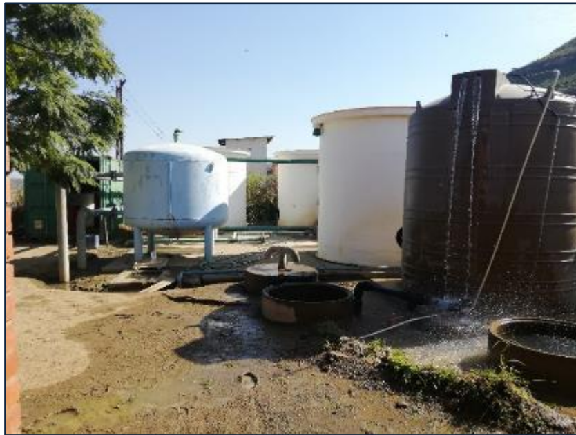
Figure 13.27 Tugela Estates Water Treatment Plant (Umgeni Water 2019).
