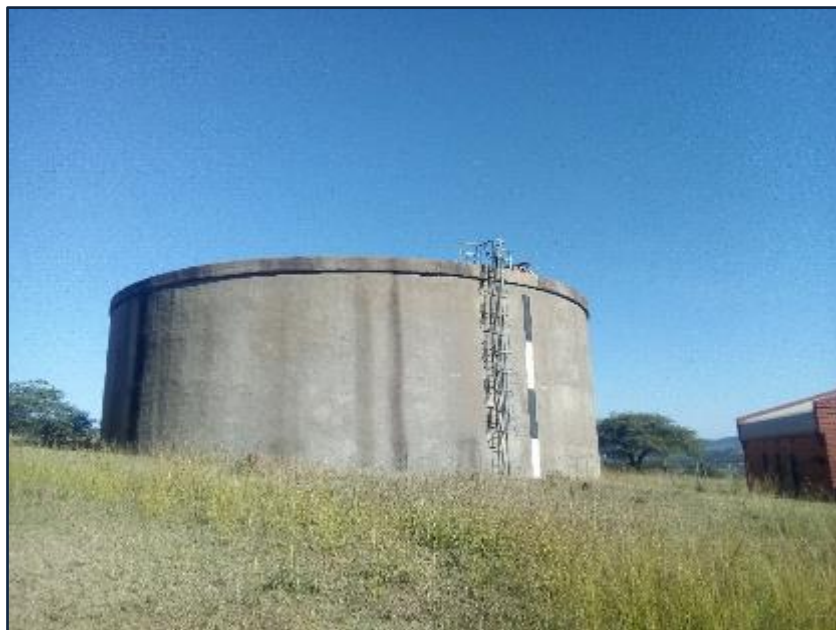
Figure 13.43 Petronella Reservoir (Umgeni Water 2019).
