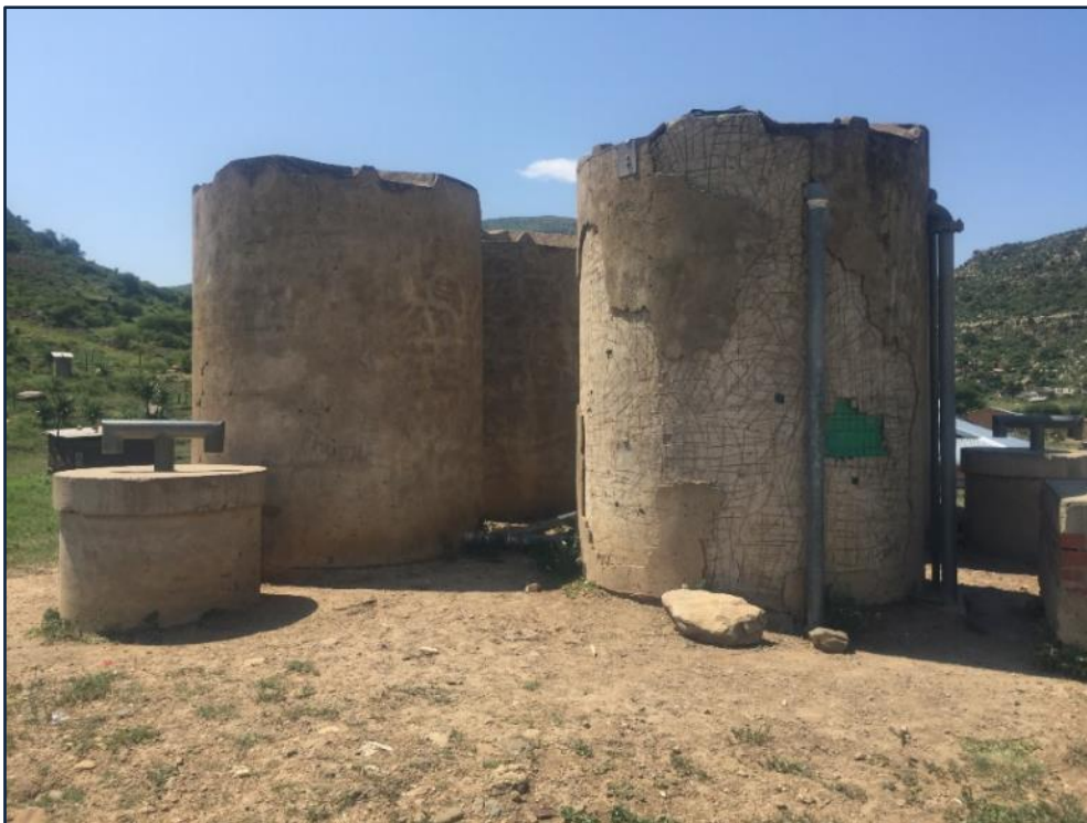
Figure 13.32 Tugela Estates Raw Water Holding Tanks (Umgeni Water 2019).
