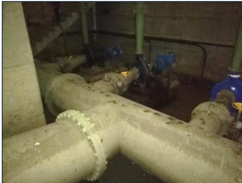
Figure 13.41 Olifantskop raw water pumps (Umgeni Water 2019).
