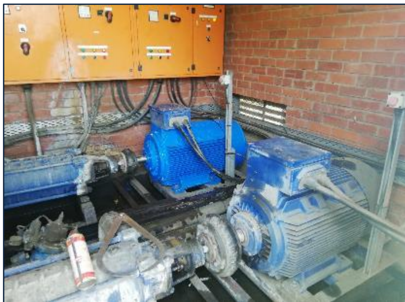
Figure 13.28 uMhlumayo Pump Station (Umgeni Water 2019).
