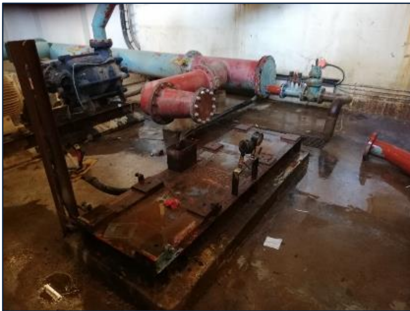
Figure 13.46 Petronella pump as of May 2019 (Umgeni Water 2019).
