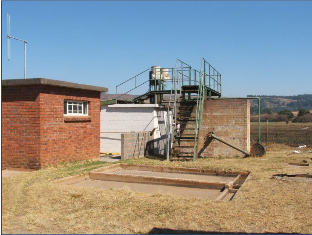
Figure 7.78 Lidgetton WTP sand wash bays with old dosing system (uMgungundlovu District Municipality 2010)
