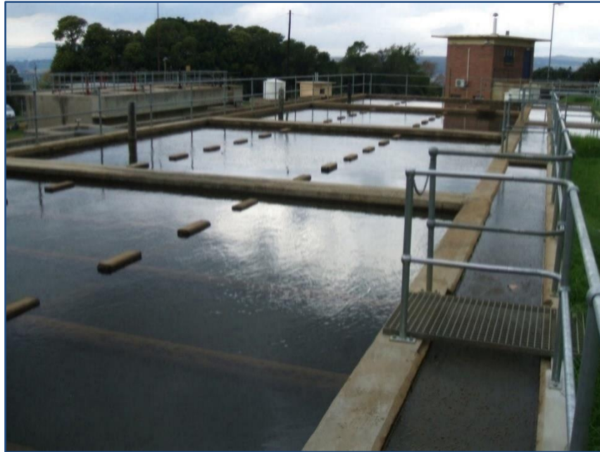
Figure 7.84 Mpofana WTP (uMgungundlovu District Municipality 2010).
