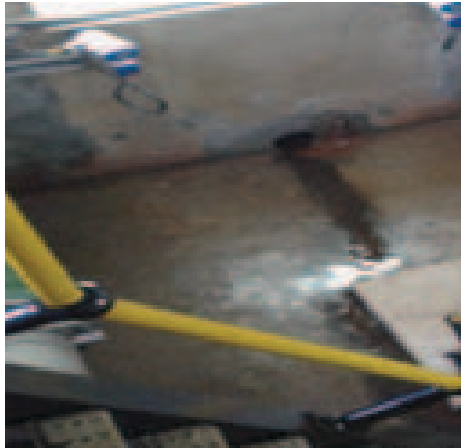
Existing flow meters at bottom of chamber
